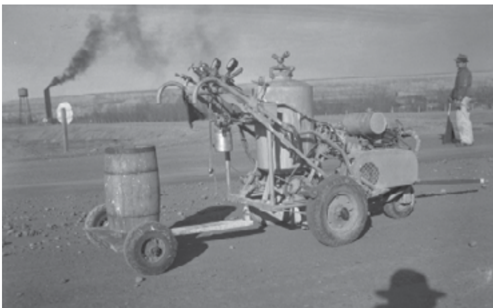
Road striping machine used at Hanford in 1944...we've come a long way!
